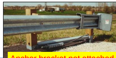
Anchor bracket not attached
